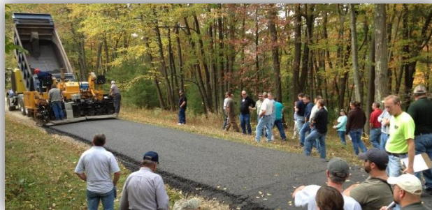
Attendees watch a paver place Driving Surface Aggregate at the 2013 Annual Maintenance workshop in Union County.
