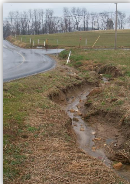
Paved roads can concentrate runoff and create erosion just like unpaved roads.
